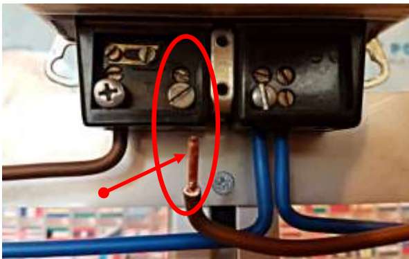
Disconnect phase wire connected to load
