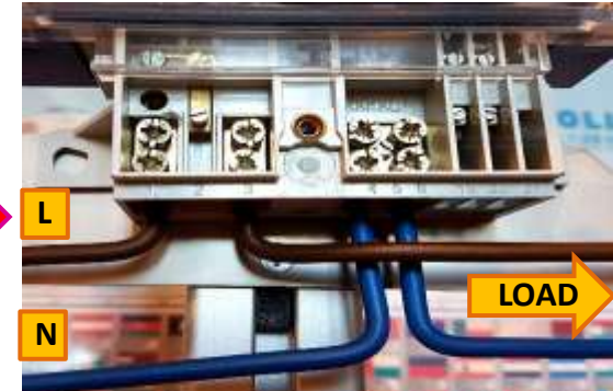
Wiring to meter terminals
